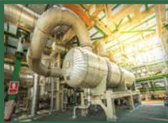
BACK PRESSURE VESSEL
